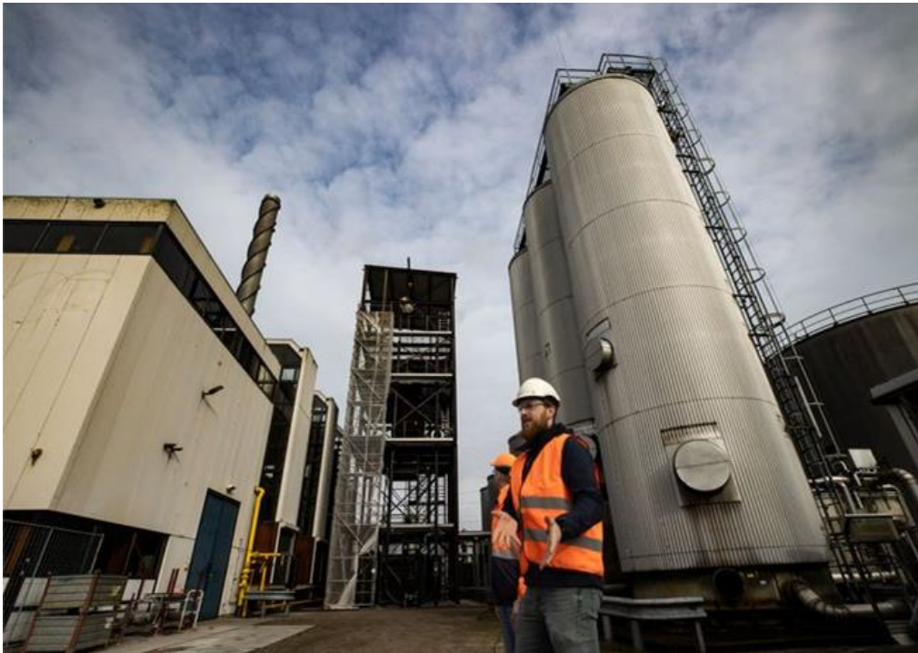
2 nd gen. combustion equipment test by RIFT at Ennatuurlijk district heating, 1 MW
