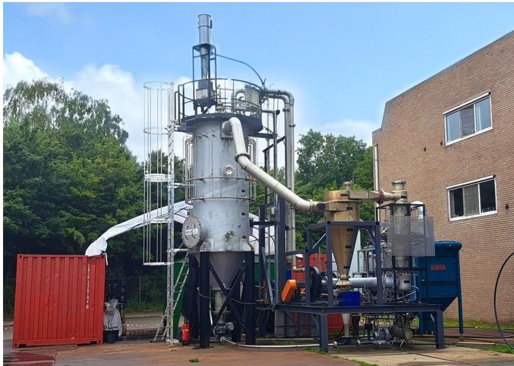
2 nd gen. combustion equipment pilot by Iron+ at Swinkels Brewery, 500 kW
