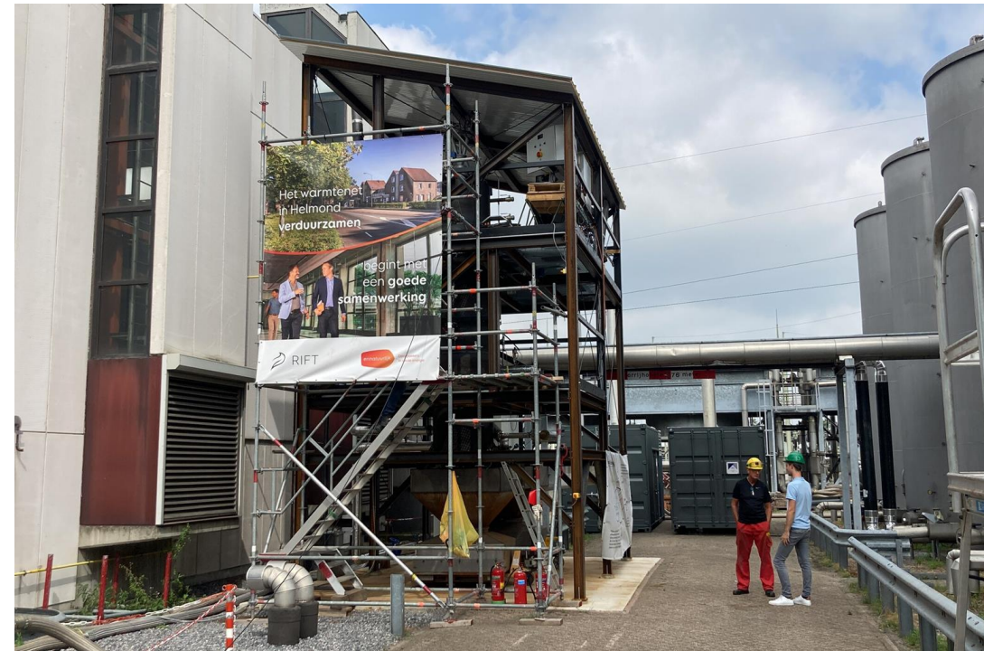
1 st gen. combustion system for district heating by start-up RIFT, 500 kW
