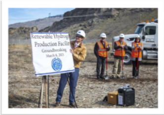
5MW electrolyzer and tube trailer refueling station in East Wenatchee for Douglas County PUD
